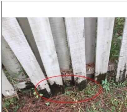
Wood deteriorating on the fence line
