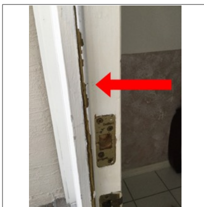
Weather Stripping on front door needs to be repaired/replaced
