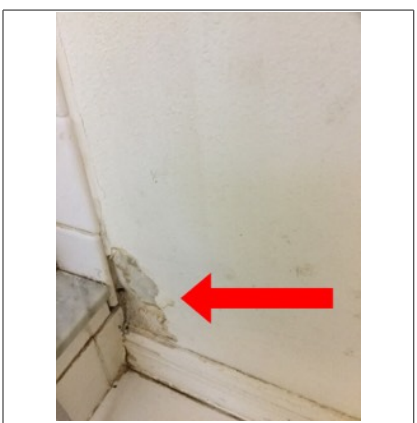
Moisture has caused this cracked drywall. Moisture reading at 95%
