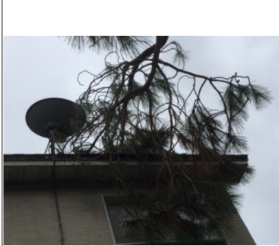
Tree branch encroaching rear roof line
