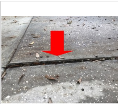
1/4 inch settlement lift on driveway
