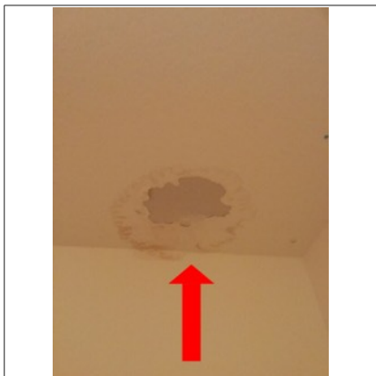
Moisture stain on ceiling in second bedroom
