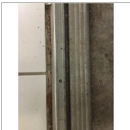
Slither of tile missing at sill plate
