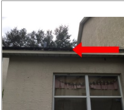
Shingle granules are beginning to separate
