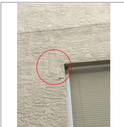
Crack side of window (Dining Area)
