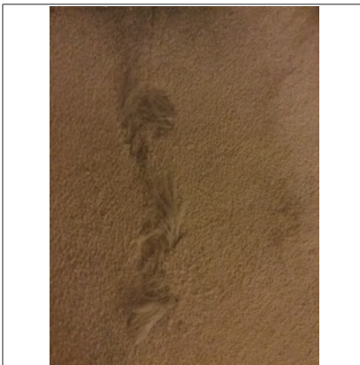
Torn carpet at entrance to Master Bedroom
