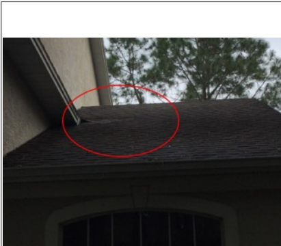
Roof appears to have had some repair work done. Also some of the shingles are cupping.
