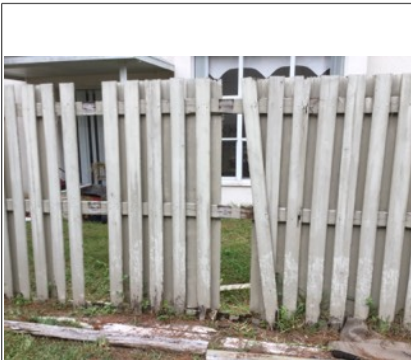
Missing Wood boards on the fence and some of the boards are deteriorating
