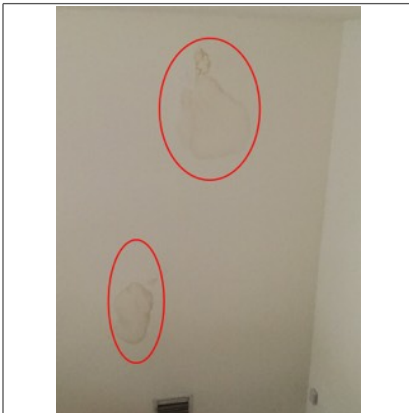
Multiple Moisture Stains above stair well
