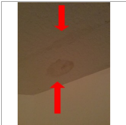
Moisture Stains on Ceiling to the left of Master Bedroom Entrance
