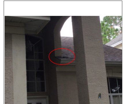
Pretty significant cupping of tiles. Evidence of leak (Dry Moisture Stains in Living Room)
