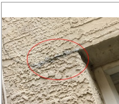
Crack above window (Laundry Room) needs to be sealed/caulked. Evidence of a leak inside property.
